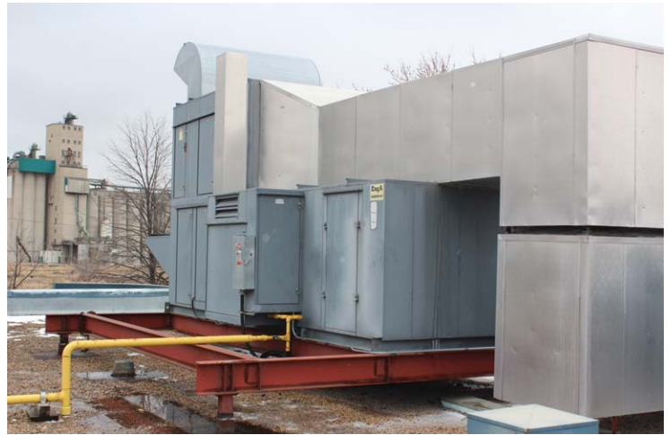
A rooftop view of the air unit at 1103 Pacific Avenue.
