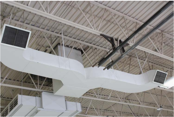
MPI's new garage air unit that helped them to significantly reduce their energy consumption.
