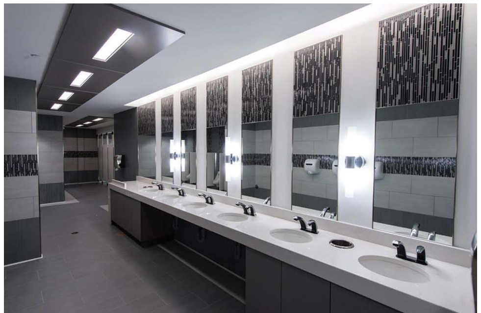
Renovated bathrooms exude a modern vibe, equipped with low flow toilets and hands-free fixtures
