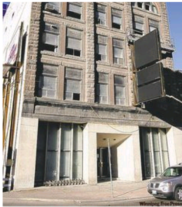
The former Ikon Office Solutions building is being turned inside-out to make way for new tenants. (KEN GIGLIOTTI / WINNIPEG FREE PRESS)
