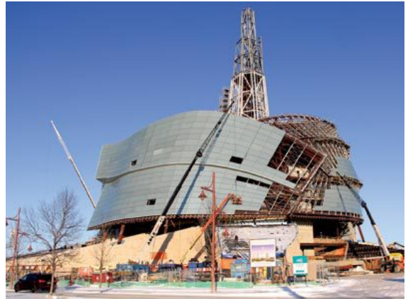
The Canadian Museum of Human Rights expects to have the base building completed by the end of this year.
